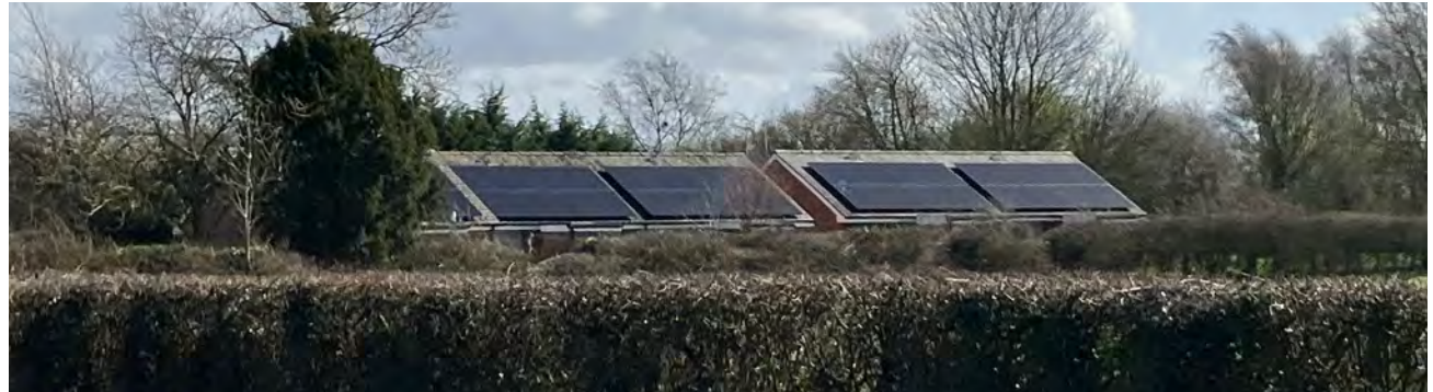
Figure 51: Solar panels on a pair of bungalows at the Apiary
