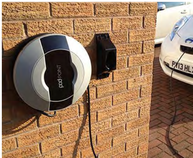
Figure 55: EV charging point
