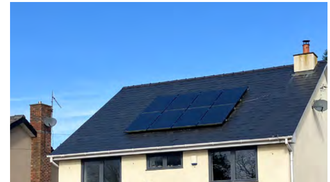
Figure 53: Solar panels on a modern property along South Road
